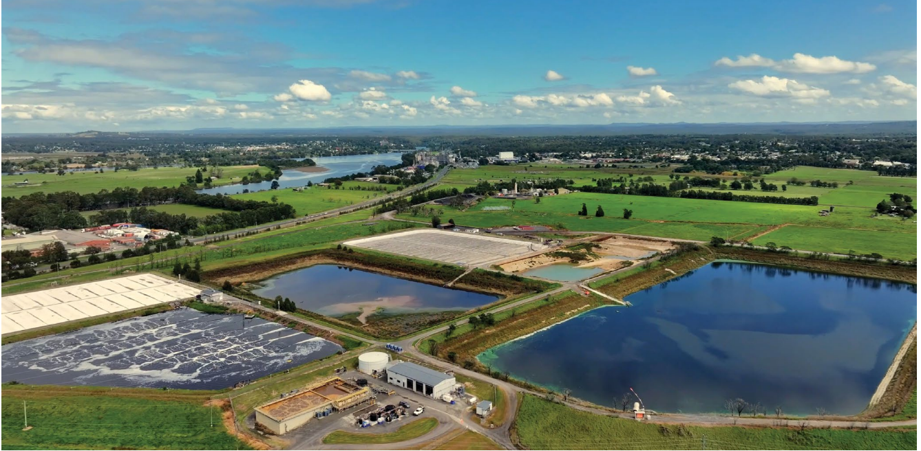
Methane captured from a wastewater treatment facility is used to power the site in Nowra, New South Wales, Australia.
