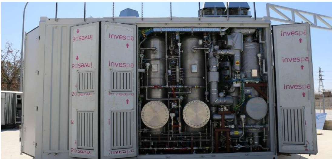
250 Nm 3 /h H 2 Natural gas reforming unit
