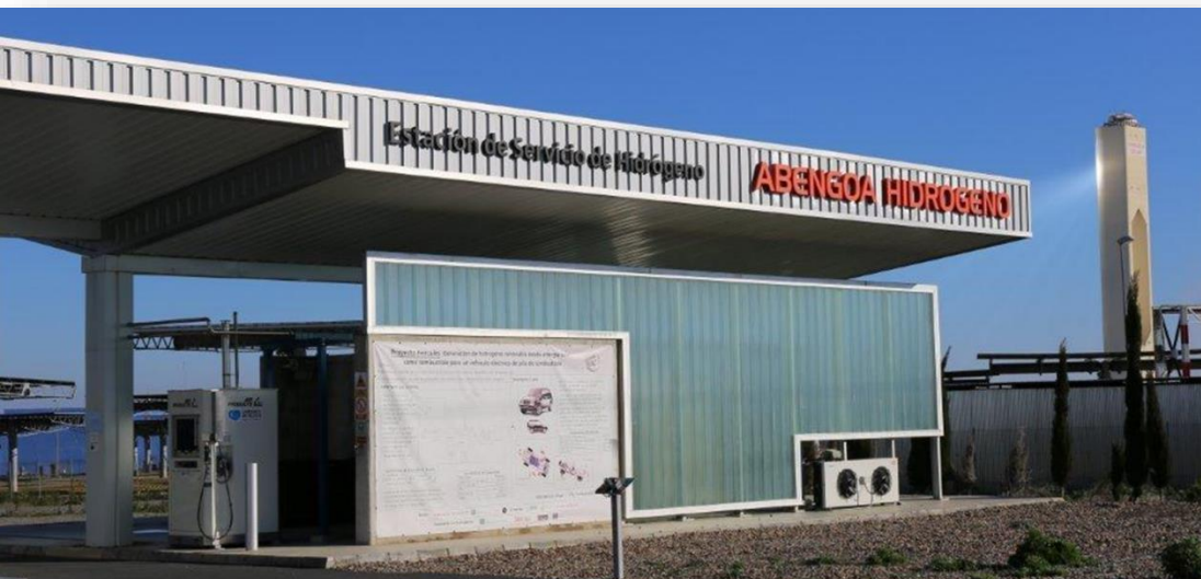
Las Columnas HRS with onsite production of 30 Nm 3 /h
